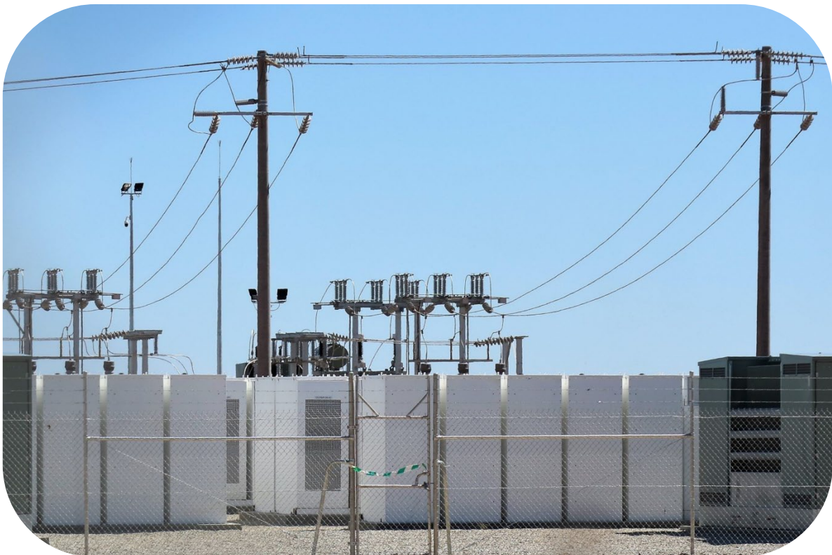
BESS on a solar farm
